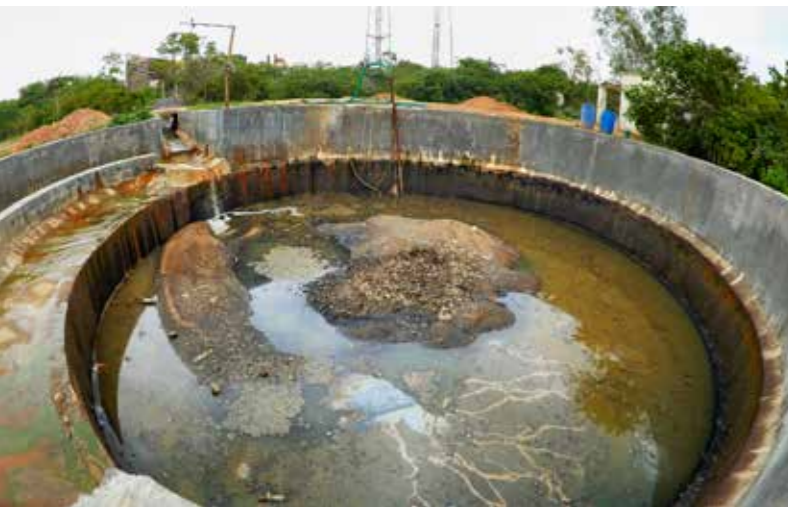
A circular effluent tank at Gadapotharam industrial estate, collecting effluents from nearby pharmaceutical factories. The tank is completely open and exposed.
